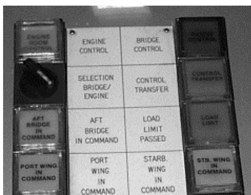
Fig. 3.13. Control transfer panel on bridge.
